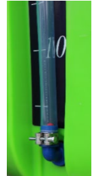
Fig. 5. Water meter the main tank
